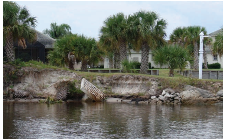
Eroded shoreline in Palm Coast
